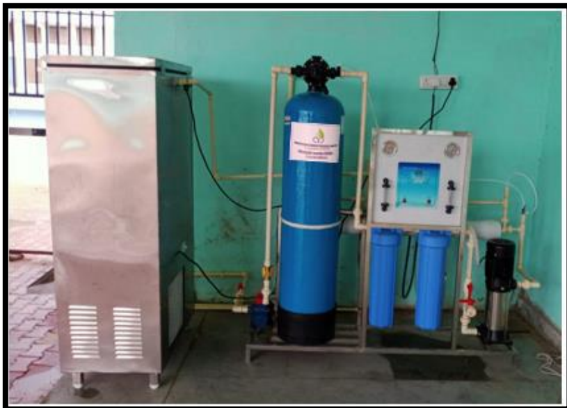
Water Purifier with Water Cooler at Education Complex School
