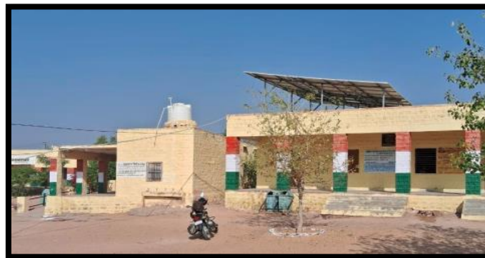
Installed Solar Panels on Govt. School
